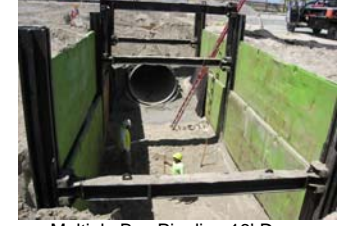
Multiple Bay Pipeline 16' Deep
